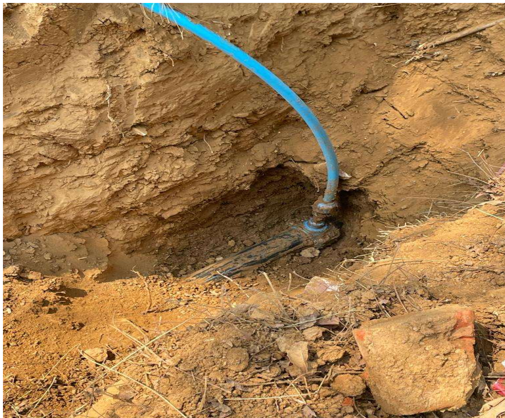
Tap connection through Flow control valves
