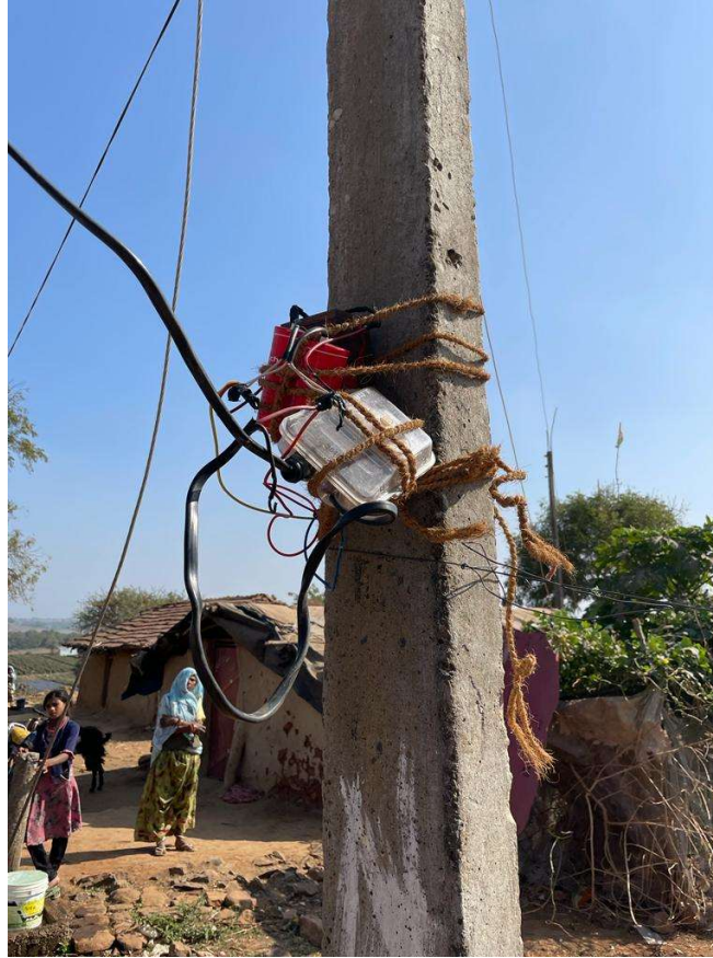
Hanging electric meter etc
