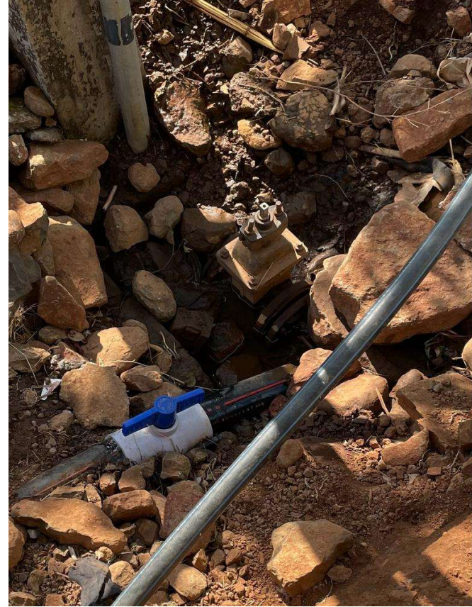
Poor sanitary conditions
