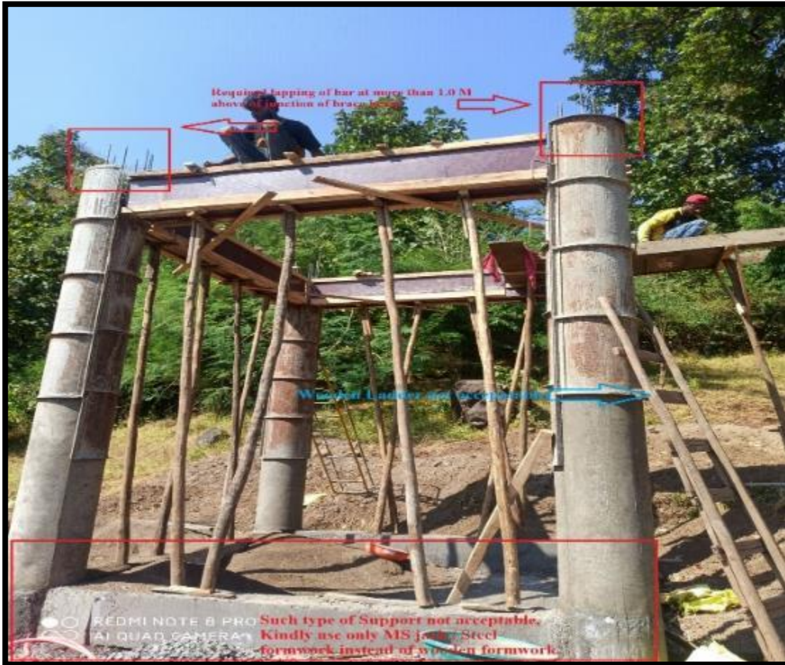
No Proper Lapping Provision for Reinforcement bars
