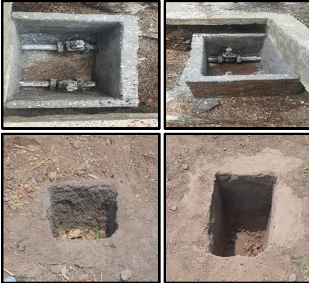
Valve Chambers Due to non-standard material use and poor skillset
