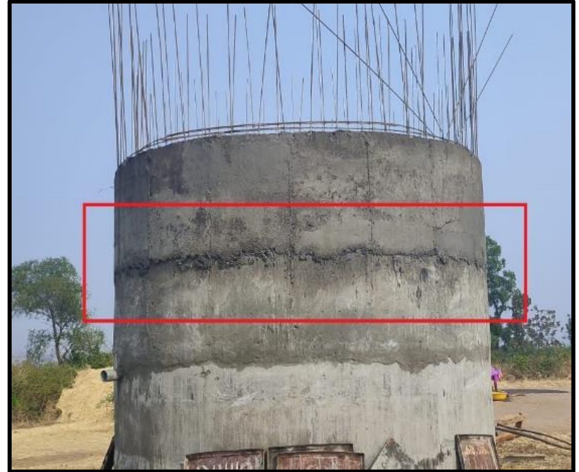
Water Retaining Structure – ESR - Concrete Joints – Leakage through Joints due to wrong practices of concreting, compaction and not using Water stopper.
