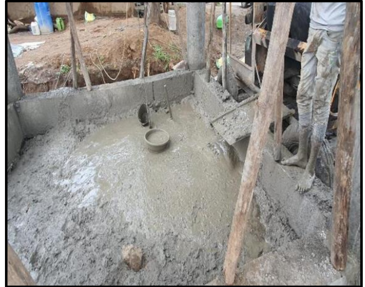
Concrete Mixing – Unregulated Mix Proportions, Mixing on ground instead of MS Tray, Use of Volumetric Mix.
