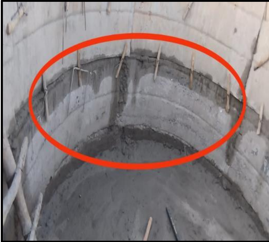
Concrete Joints - Undulations in Surface - Due to poor quality of formwork material
