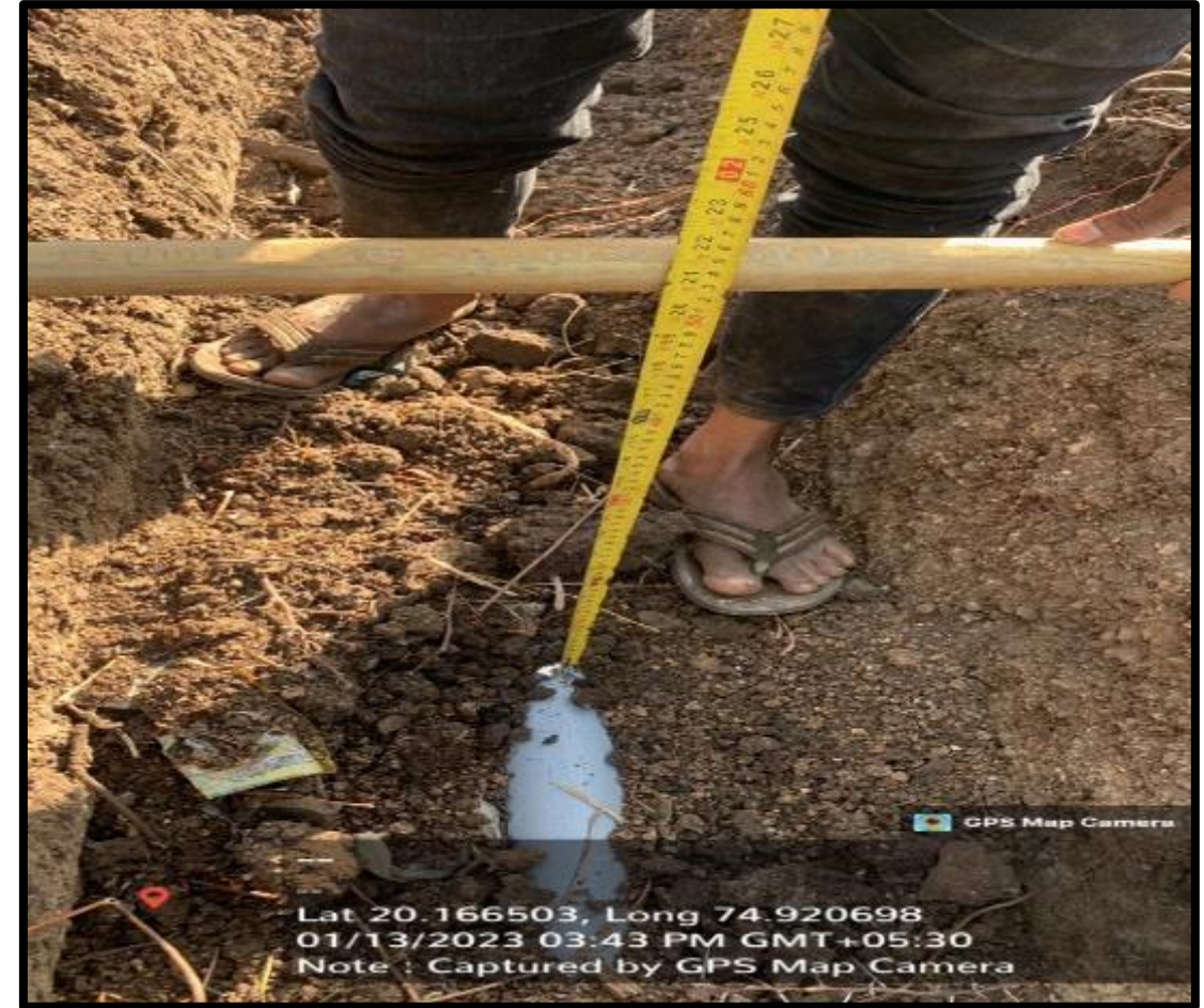
Insufficient excavation depth / soil cover for Piping work resulting in insufficient cushioning for Pipes.
