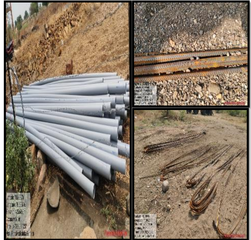
Improper Stacking of material
