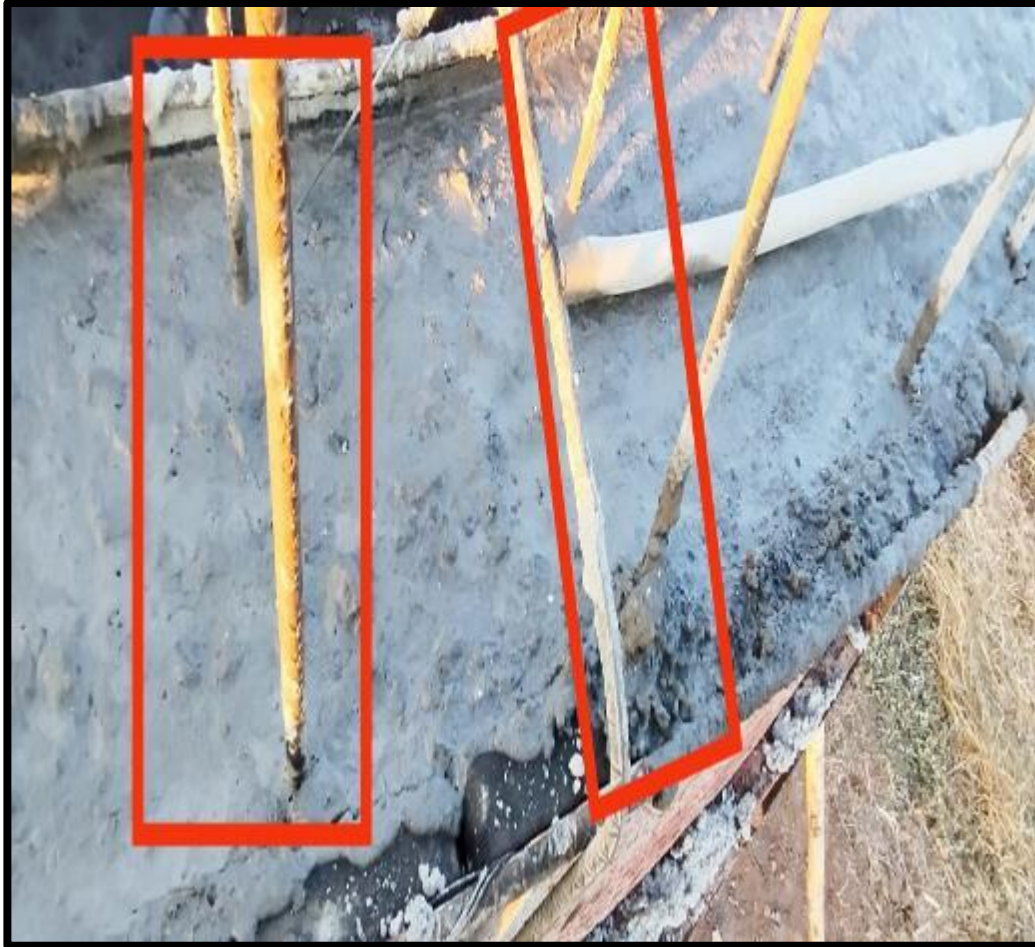
No Proper or sufficient Concrete Cover for Reinforcement
