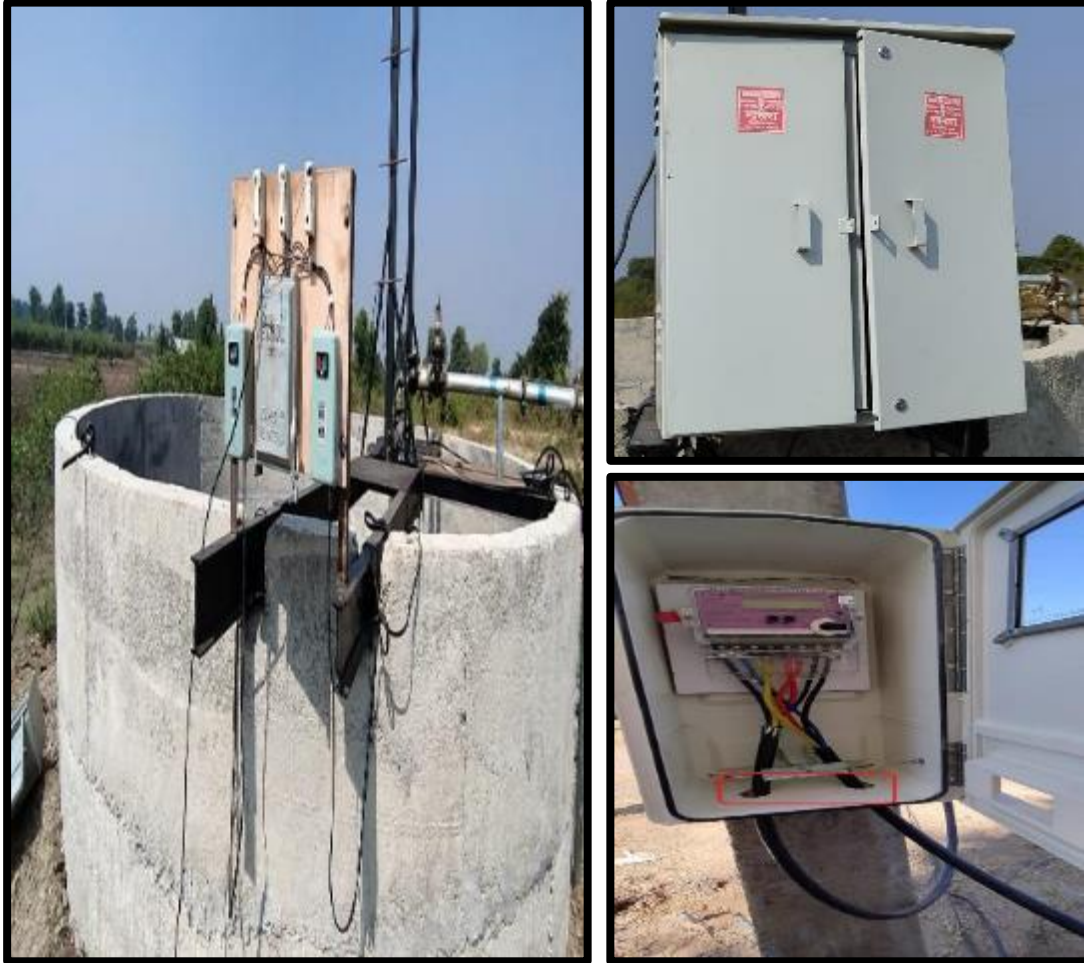
Required enclosed panel board / DB board with proper Gland for cabling work
