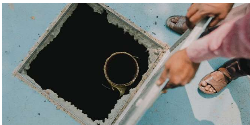
Abandoned borewell converted into recharge structure
