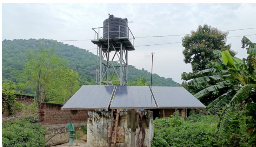
Figure 10: Solar based PWS in PVTG village | Source: RWSS Odisha
