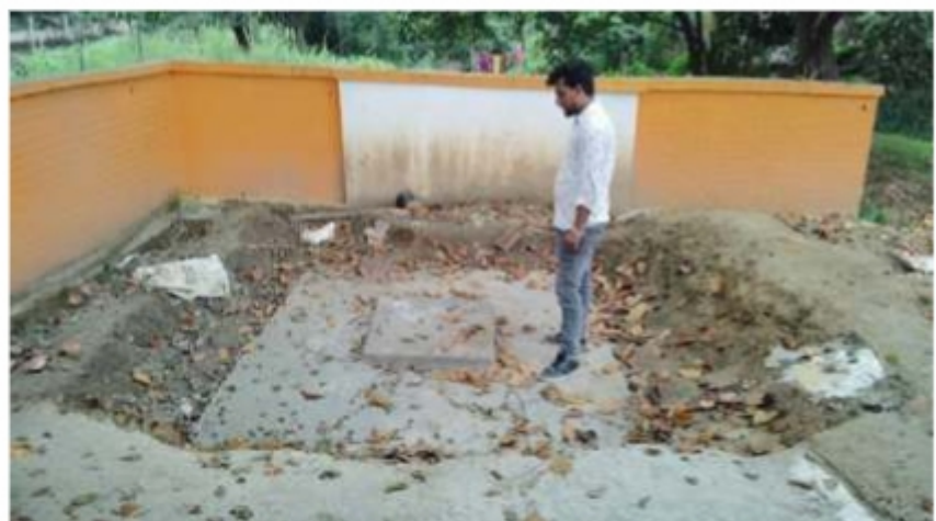
Figure :59 | Community Soak pit-a step towards water source sustainability | Source: DWSM Bahraich, Uttar Pradesh
