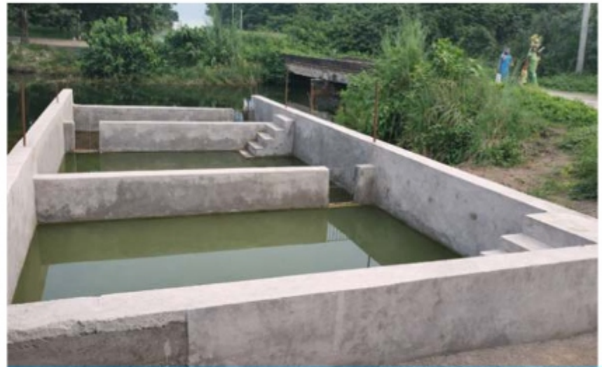
Figure 63: Waste Stabilization Pond (WSP) | Source: DWSM Raebareilly
