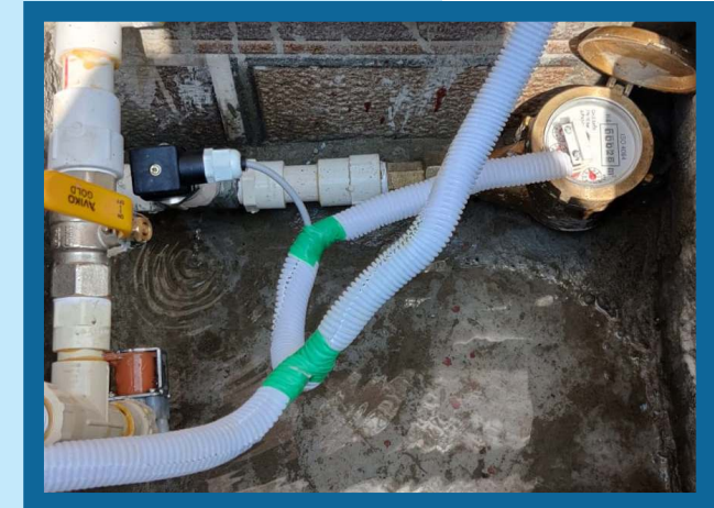
Water quality, pressure & flow sensors at consumer end
