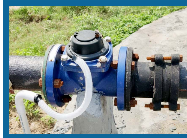
Flow meter sensors installed at water source
