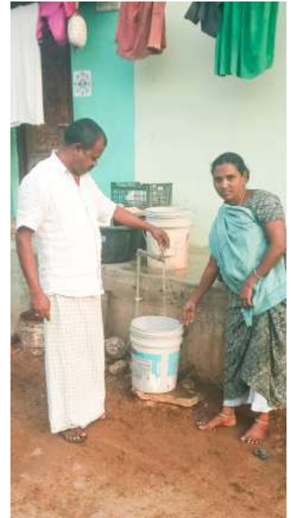
FHTCs transforming village life with convenience and dignity | Source: PHED, Andhra Pradesh
