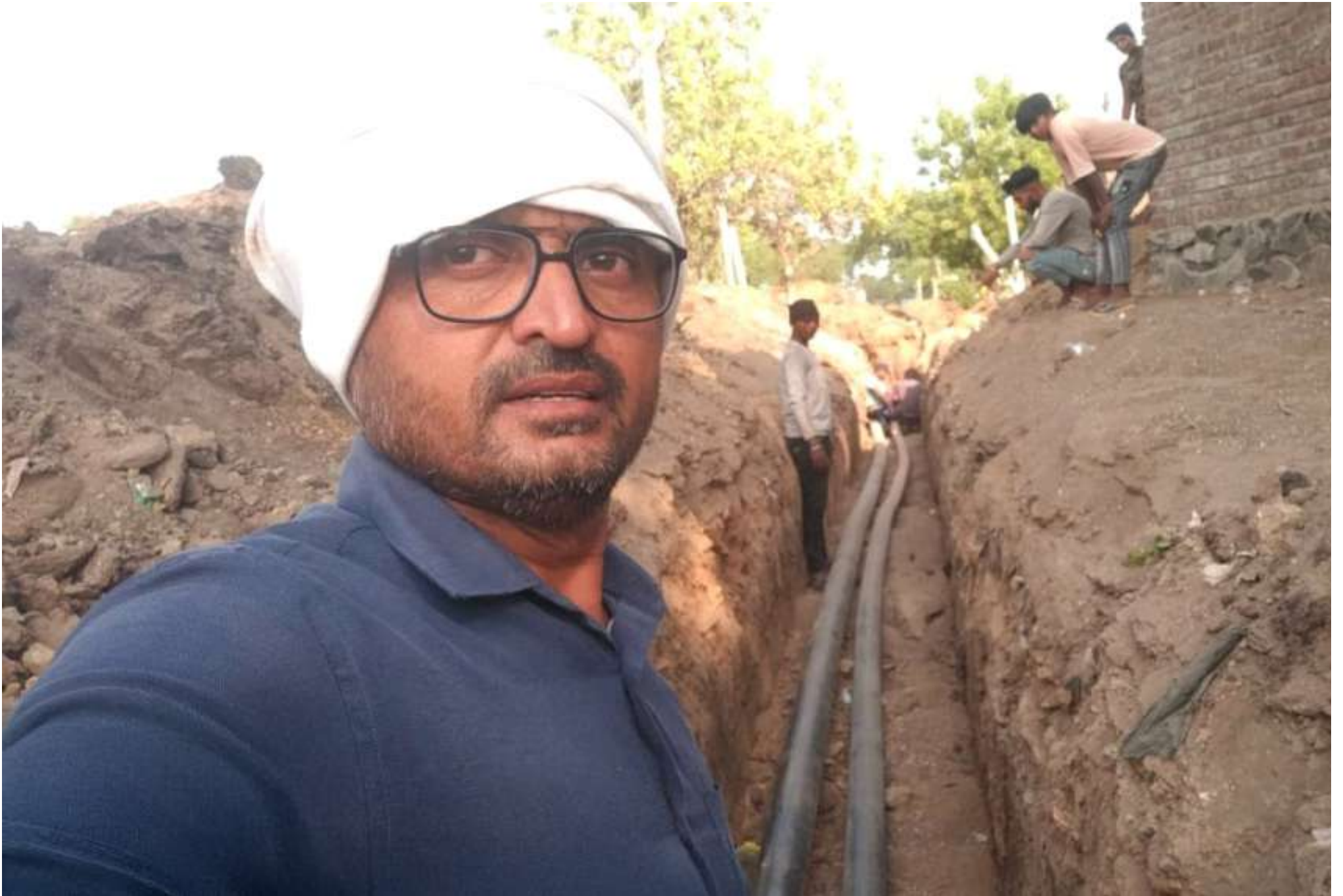
Shri Manoj overseeing the installation of distribution pipelines under JJM | Source: PHED, Maharashtra
