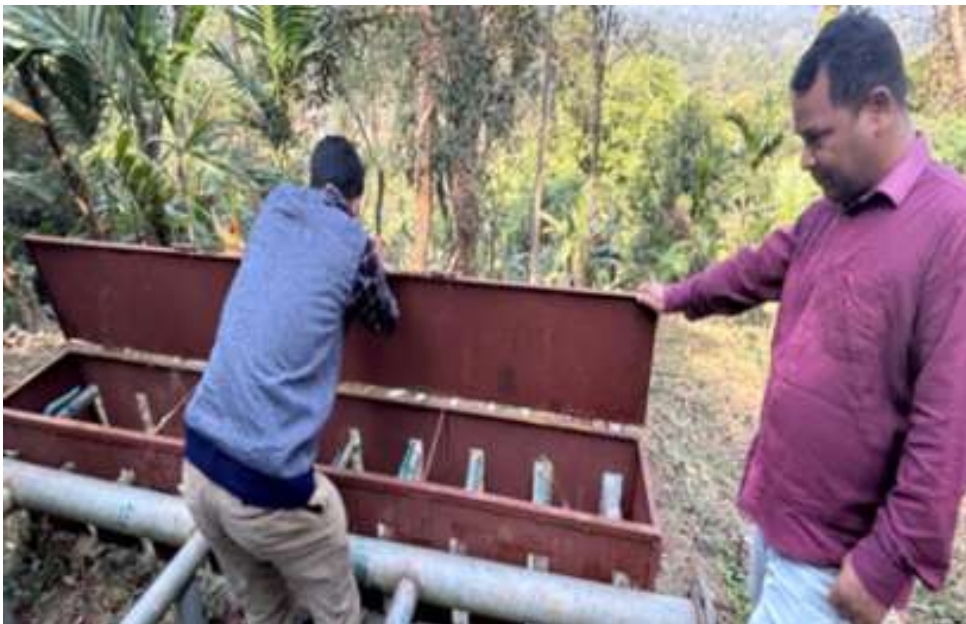
Images showing the inspection of Distribution pipes by the VWSC members | Source: PHED Meghalaya
