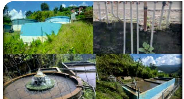
JJM assets in Zokhawthar village, Mizoram transforming the lives of people
