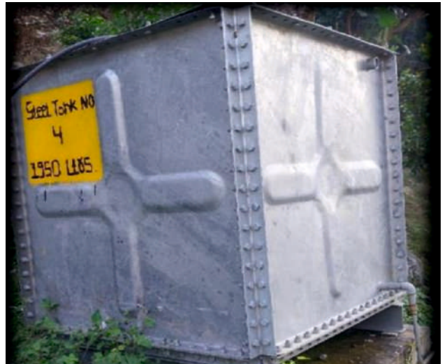
Storage tank constructed under the Jal Jeevan Mission Source: PHED, Sikkim
