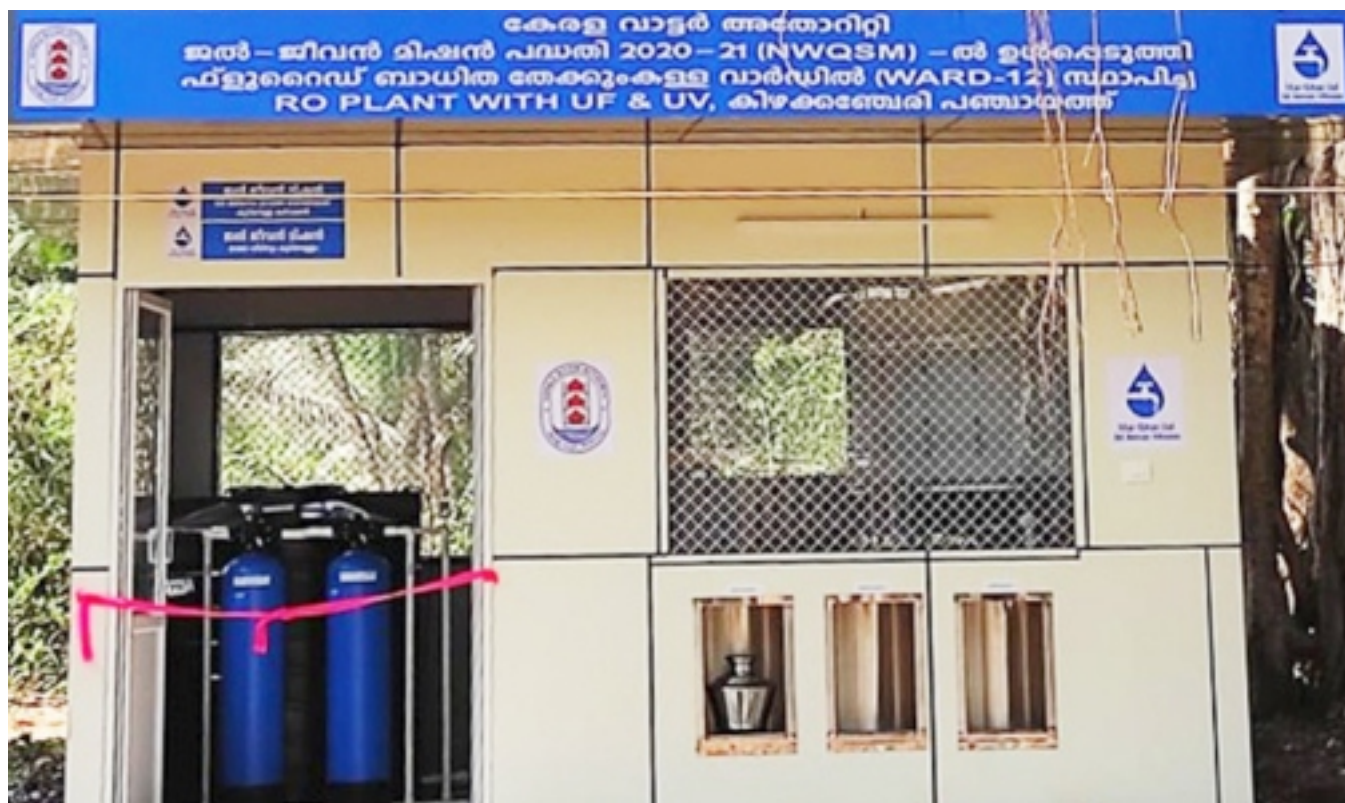
Community water purification plant in Kerala
